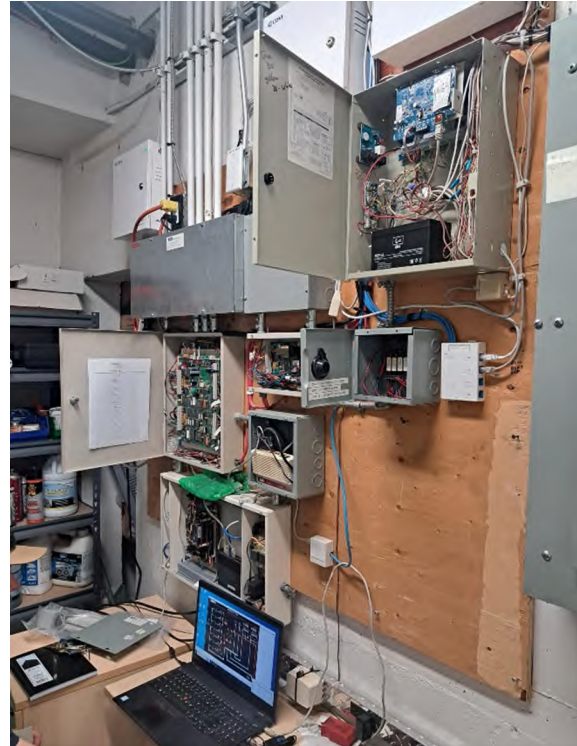
City Hall Climate Controls
